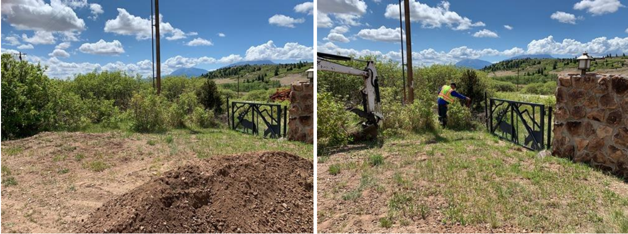
Location of Emergency Access Gate. Existing gate will be expanded to East (Left in Picture)
