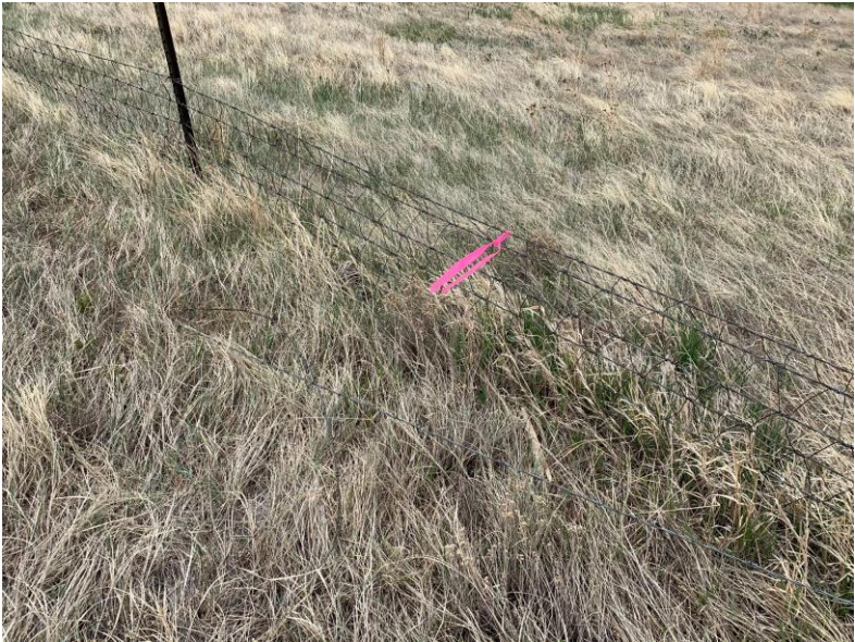
Typical damage to Southern Fence Top strands of barbed wire are down
